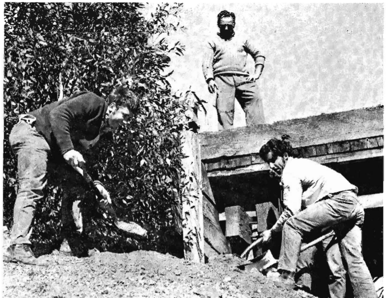
Members of Ballarat Works Gang No. 2 are currently working on bridges between Ararat and Maryborough. See here digging around sheeting on a bridge near Dunneworthy are (left to right) Bill Cocking, Bob Booth, John Rivett and Geoff Garter (obscured).
