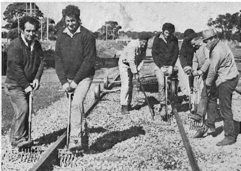
Track gangs No. 5 (Dunkeld) and No. 6 (Moutajup pictured recently at work on the Ararat-Hamilton line near Dunkeld.
