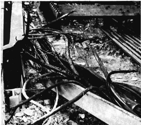
At E Box, one of several locations where lead sheathed cables were burnt through by the current.
