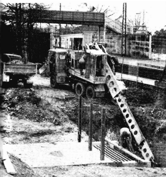
subway, at the Box Hill end of the station will replace the existing platform. The existing platform will be converted to an island platform. Work at the Union Road end, will be started shortly.
